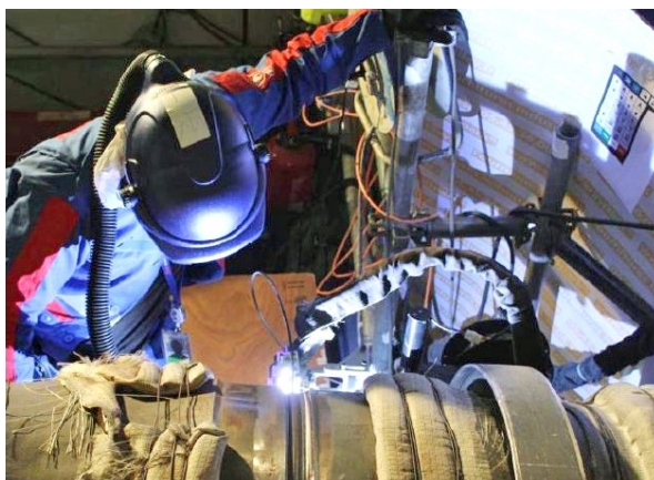
Implementation of the orbital TIG process –weld on the main secondary system
